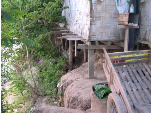
Many of the homes in the village are in danger of slipping of the river bank.
