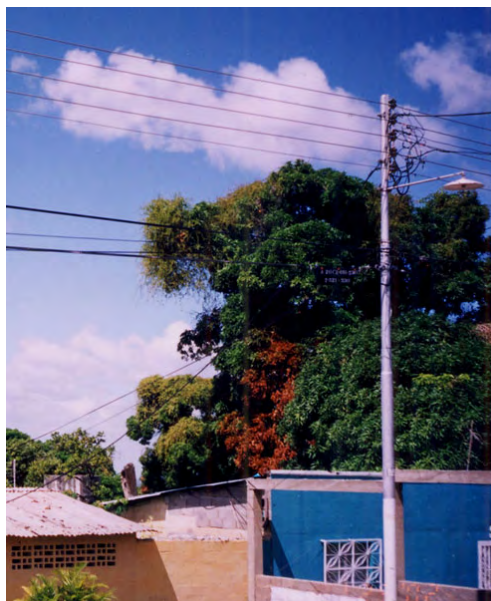
the energy pole seen here is still accessible for maintenance
