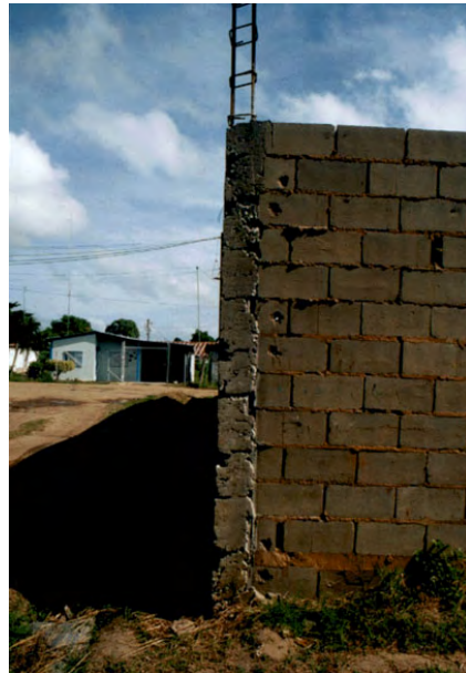
image 5: cold joints in poured concrete
