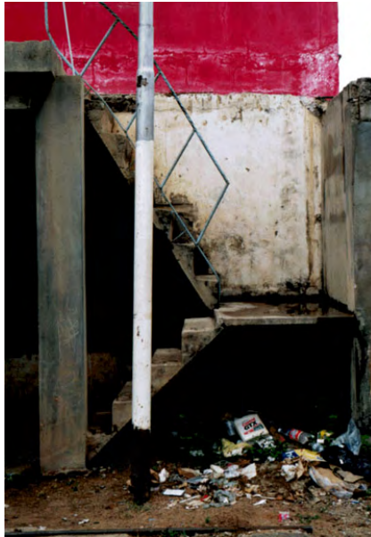
image 6: minimal concrete thickness
